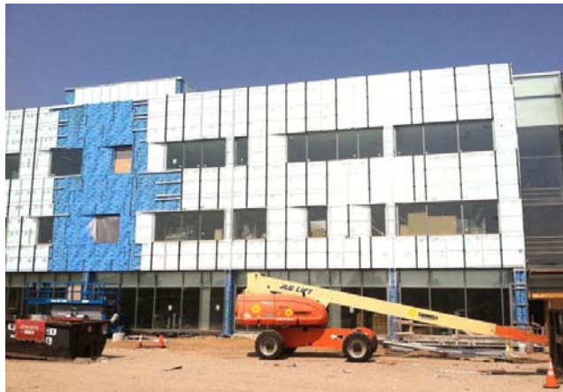
Nearing Completion: Nassau Community College Life Sciences Building LEED Gold Goal: Cannon Design, Architects; Sustainable Design Collaborative LLC (Green/LEED)
